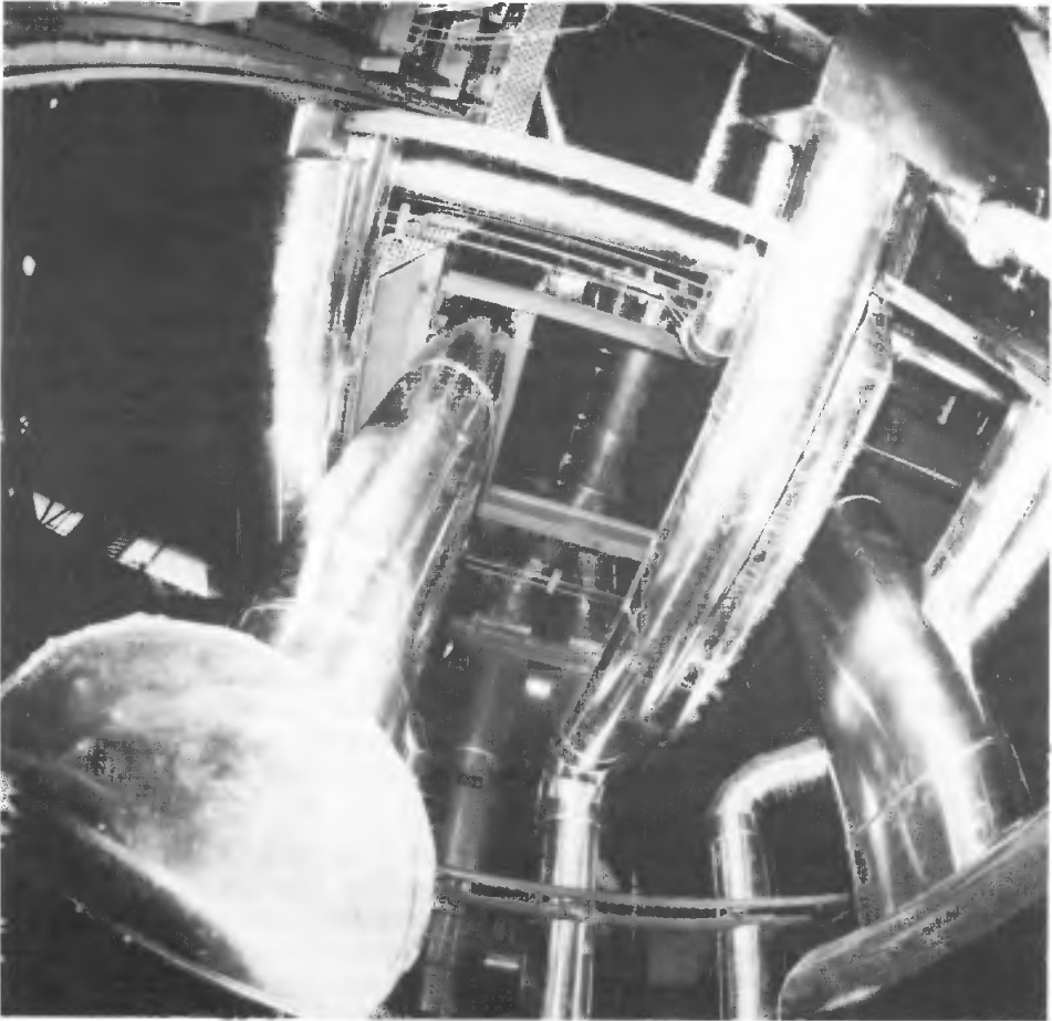
High-pressure hydraulic test rig (Light water reactor testing programme) (Reactor safety project, Ispra).
