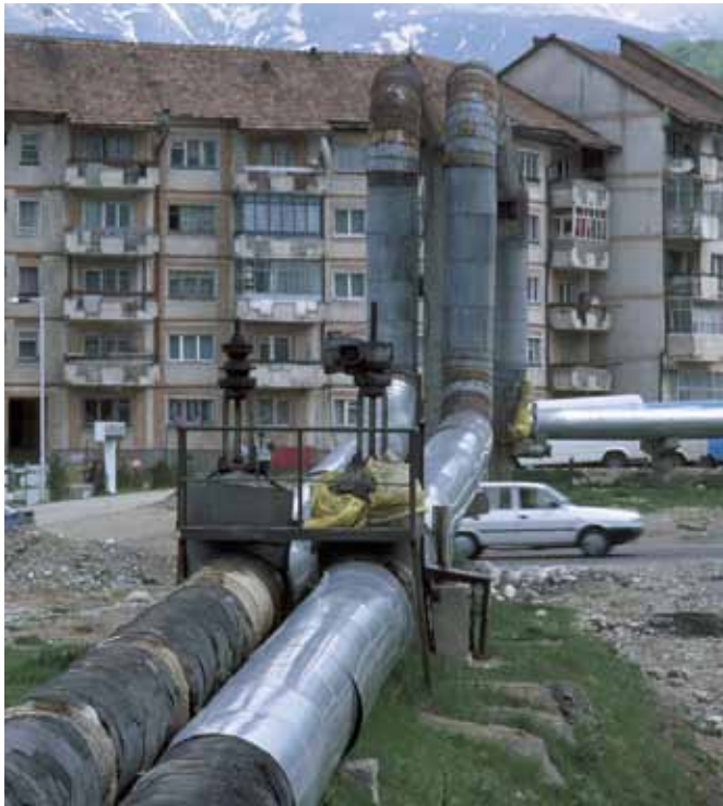
Town heating pipes, Romania
