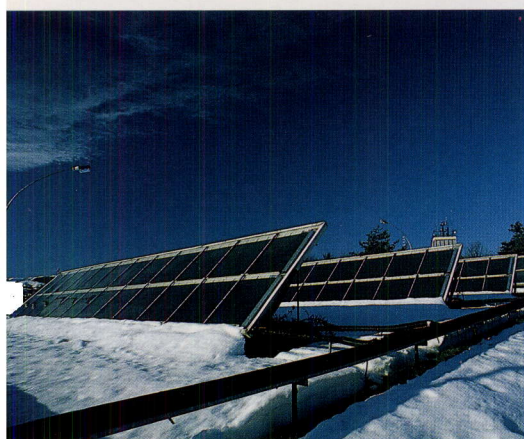
Figure 71: An array of solar collectors used for seasonal storage
