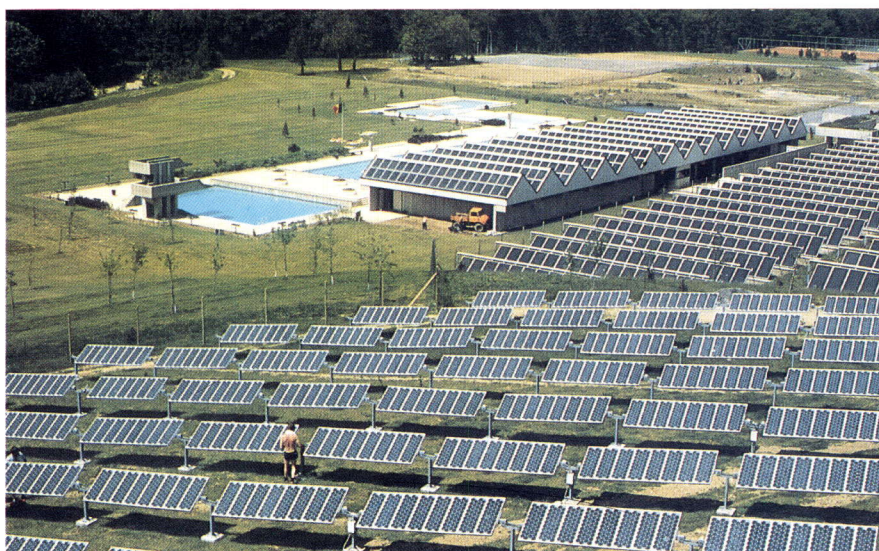
Figure 76: Solar-thermal panels heat a swimming pool in Chevetogne, Belgium, while its electric supply is provided by photovoltaic modules.
