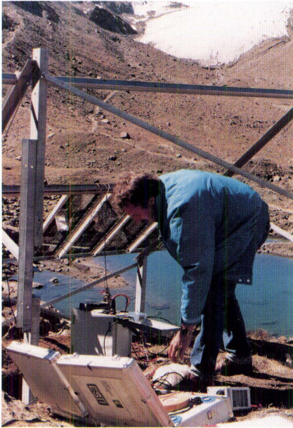
Figure 74: A member of the ESTI team during on-site measurements of a photovoltaic installation in the Alps (altitude 2610 m)
