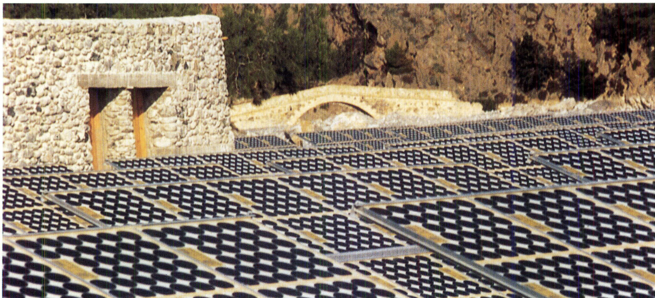
Figure 87: The 50 kW PV plant at Aghia Roumeli (Crete) is followed by ESTI using on-site power measurements and data from monitoring.
