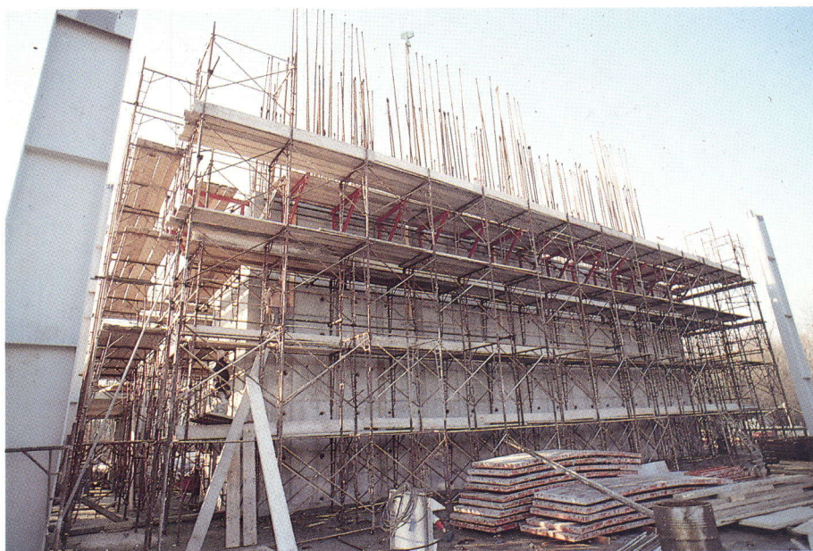
The reaction wall test facility under construction on the Ispra site of the JRC.
