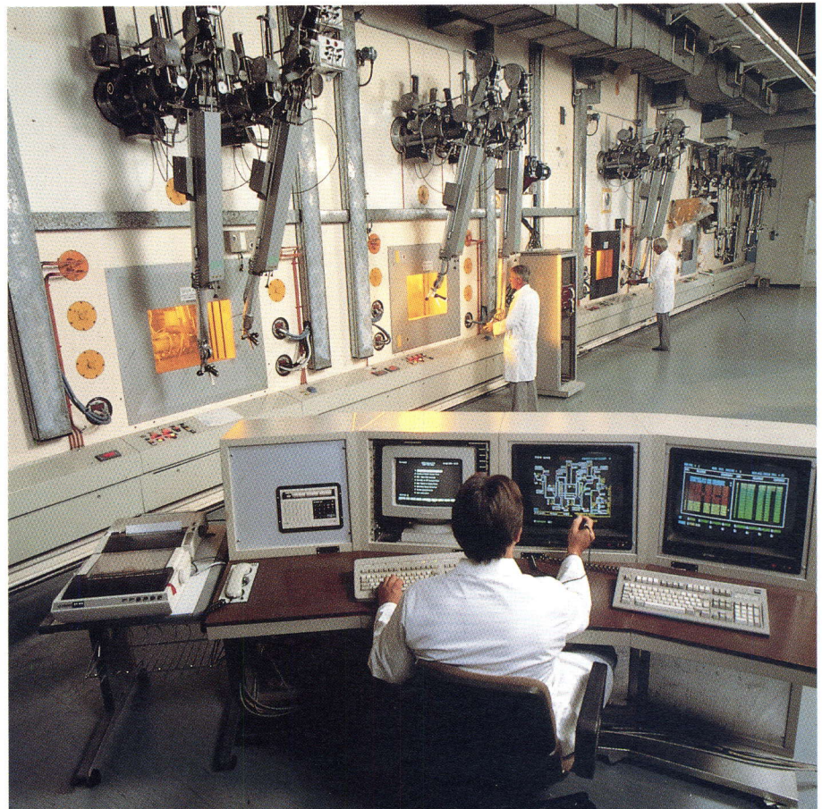
Overall view of the PETRA facility showing the three main hot cells and the Process Control System (PCS)
