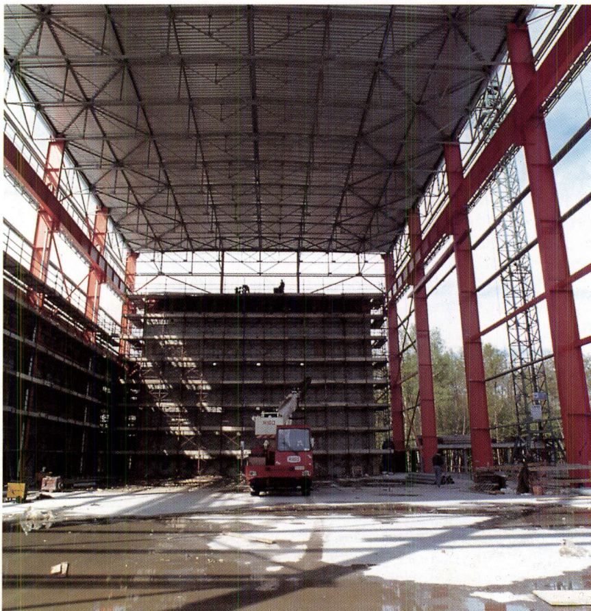
Reaction wall facility under construction at Ispra for testing of large-scale models of structures
