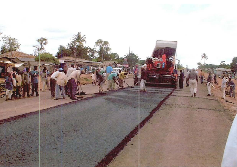
Road building in Nyanguge, in the Mwanza region of northern Tanzania, close to Lake Victoria.
