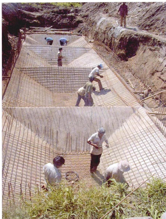
Building of sewerage system in the municipality of Chimoré in the tropic of Cochabamba, Praedac programme.
