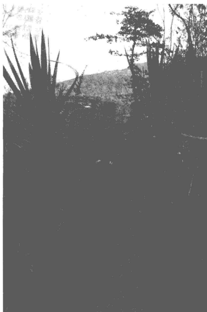
A trench being dug to take a water pipe. MIDP uses voluntary labour to undertake trenching work where the local community is the main beneficiary.
