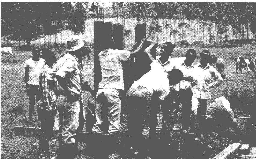
Flood control, irrigation and drainage construction works... the active involvement of several thousand local people has been perhaps the greatest achievement of the Nyanza Rice Project.
