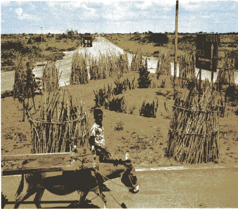
Somalia : the resurfacing of the road leading from the main region of agricultural development to the capital.
