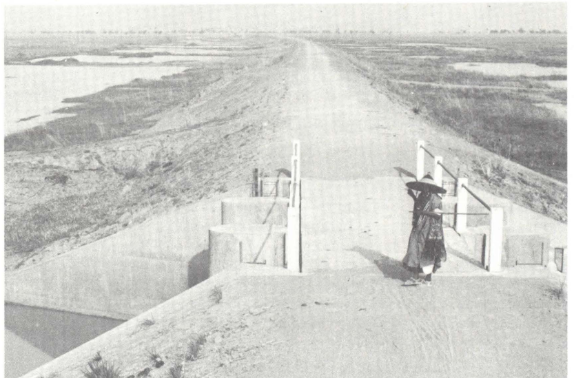
In Mali the flooding of the rice fields is carried out by a system of dykes.
