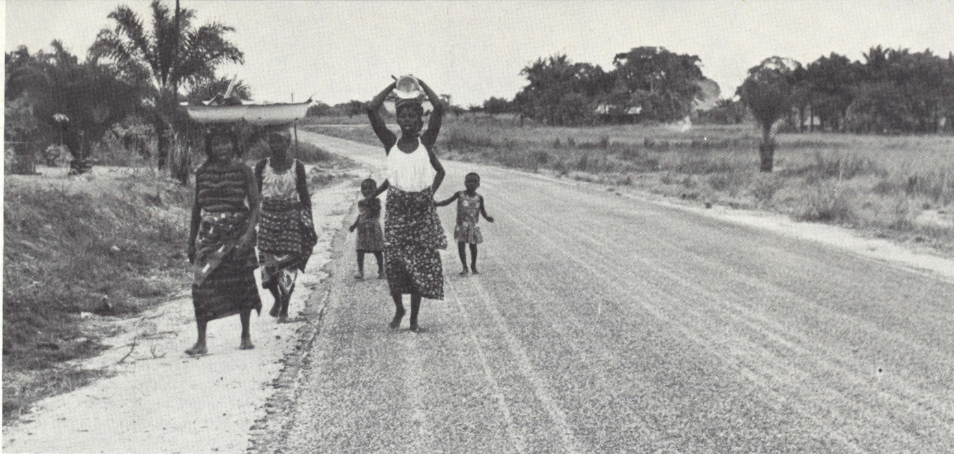
The EDF surfaced this road from Kinkala to Brazzaville to speed up market supplies into the Congo capital
