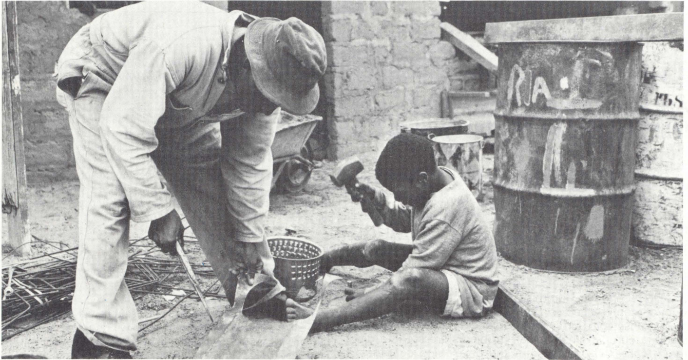
Starting a family business — building a house can lead to other initiatives
