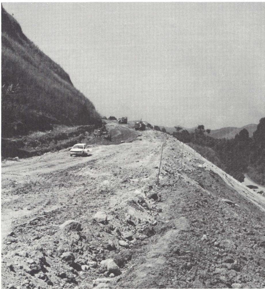
Construction of the Bafoussam-Bamenda road: building up a difficult section of the highway at the 35 kilometre point
