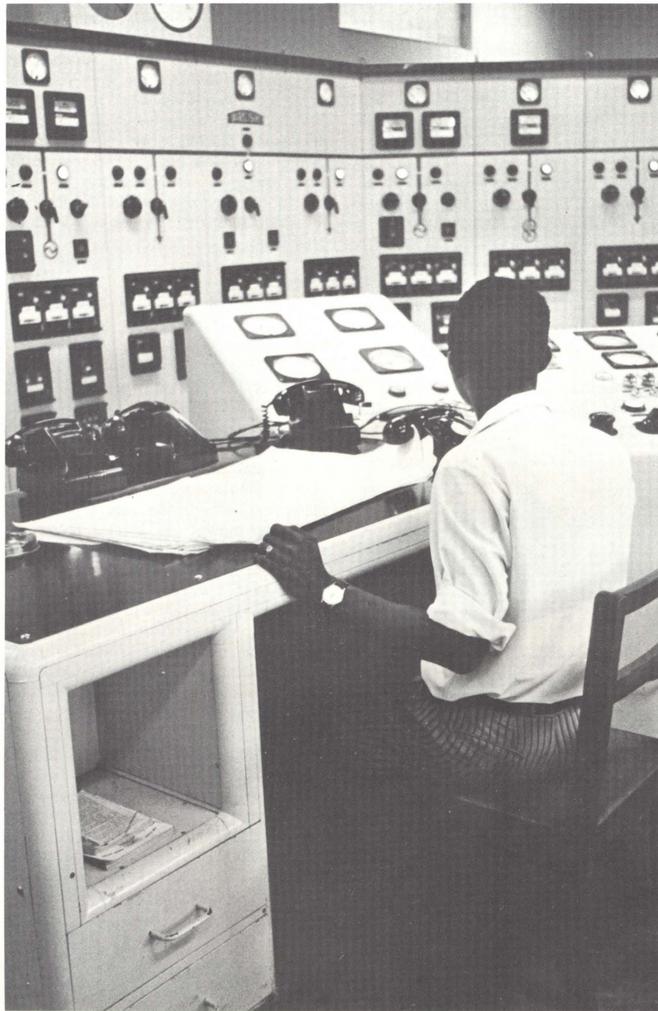
Control room of a power station in Sierra Leone co-financed by the World Bank and ABEDA
