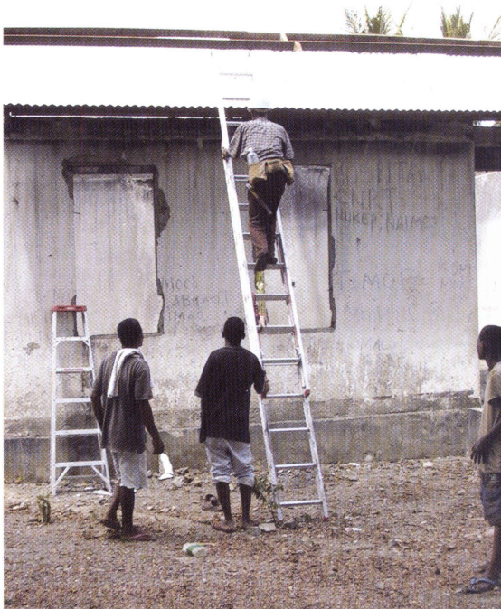
Workers from a local NGO rebuild a house destroyed during the war.
