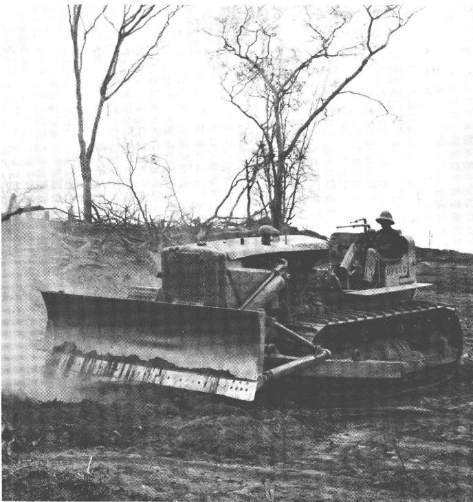
Most of the roads financed by the EDF form part of a trans-African network, such as the N'Gaoundéré-Garoua road in Cameroon, seen here under construction...
