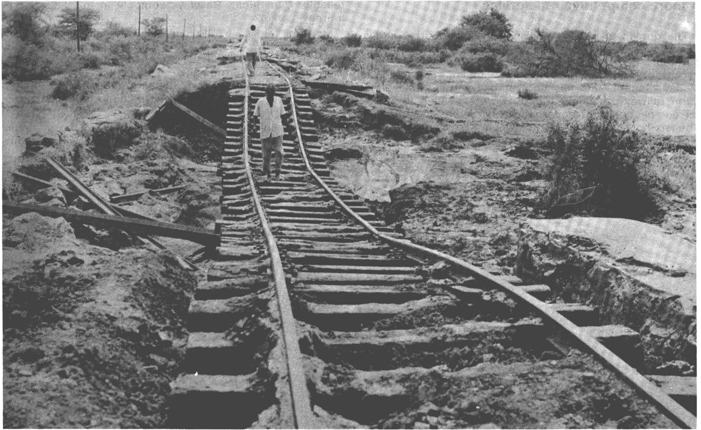
Damage caused by rain to railway track in the west of Sudan
