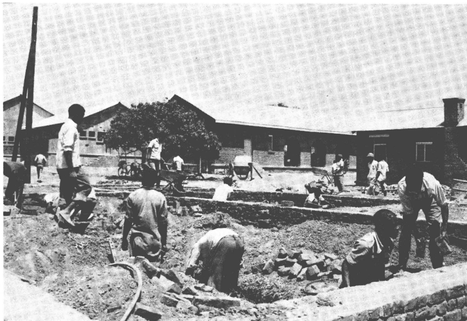
Extension of Katete hospital in the east of Zambia, one of the countries where Dutch aid is concentrated
