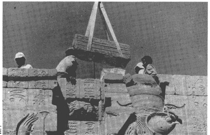
On the new site of the monuments, at Algikia island. One of the 47 000 stones, weighing some 12 tons, is put in place
