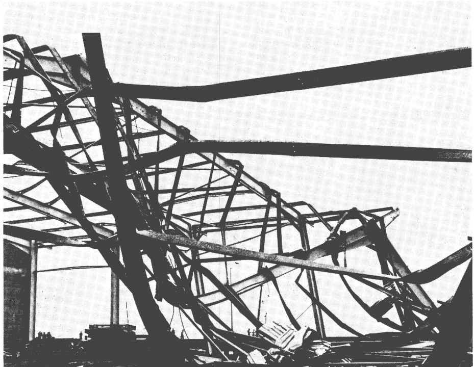
These twisted metallic beams left behind by another cyclone, David, in Dominica, bear witness to the destructive force of hurricanes
