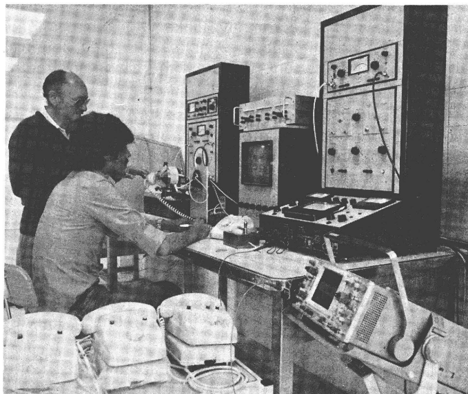
Transfer of technology: an Algerian technician, one of 3000 trained by ITT's Spanish subsidiary in 1976-80. Algeria now has its own telecommunications plant
