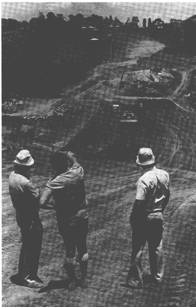
Construction of the Thuchi-Nkubu road in Kenya, financed by the United Kingdom. "A synthesis evaluation of a number of road projects funded by the ODA and other donors showed that many new roads were not being properly maintained because there were not enough trained personnel, and sometimes because equipment was not available"
