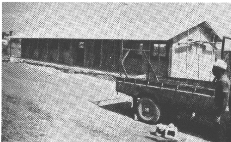
Construction of a classroom block at the Port Loko Teachers Training College
