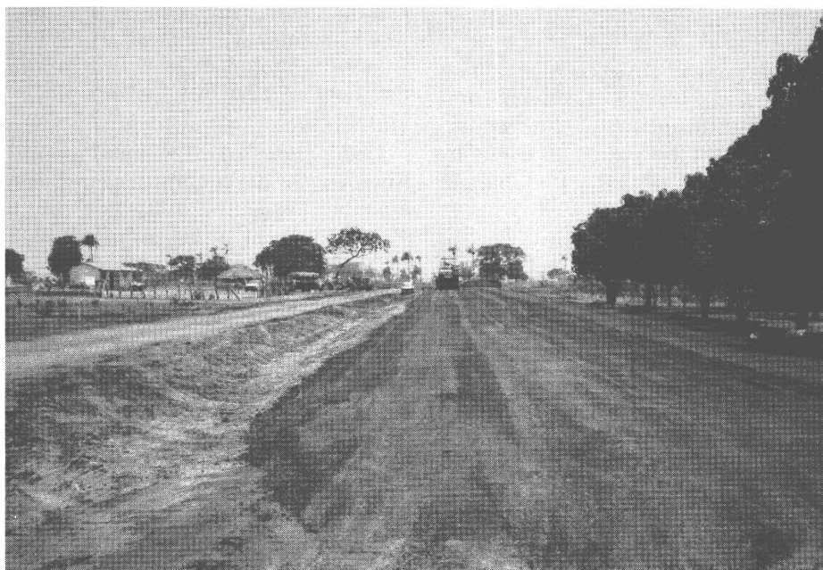
Road construction is an important element of The Gambia's share of the EDF budget
