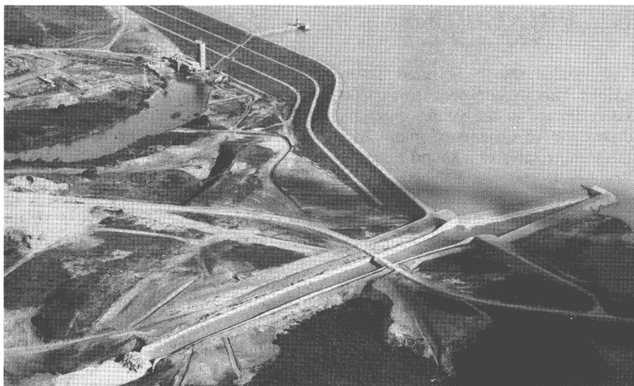
A typical example of co-financing: the Masinga dam over the Tana river, in Kenya, jointly funded by the Federal Republic of Germany, the United Kingdom, Kenya, the EDF and the EIB
