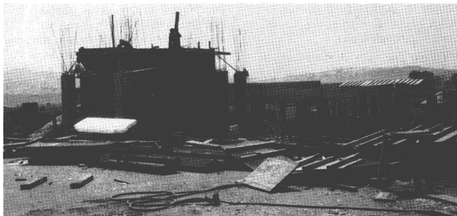
The control tower of Matsapha airport under construction. It is being financed by the EDF within the framework of regional programme for Southern Africa
