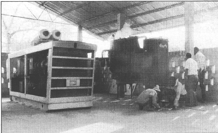
Pilot fuel-gas generator installed with CDI assistance in Gambia.
