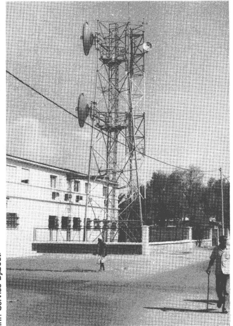
Satellite communication equipment at the Djibouti town post office.
