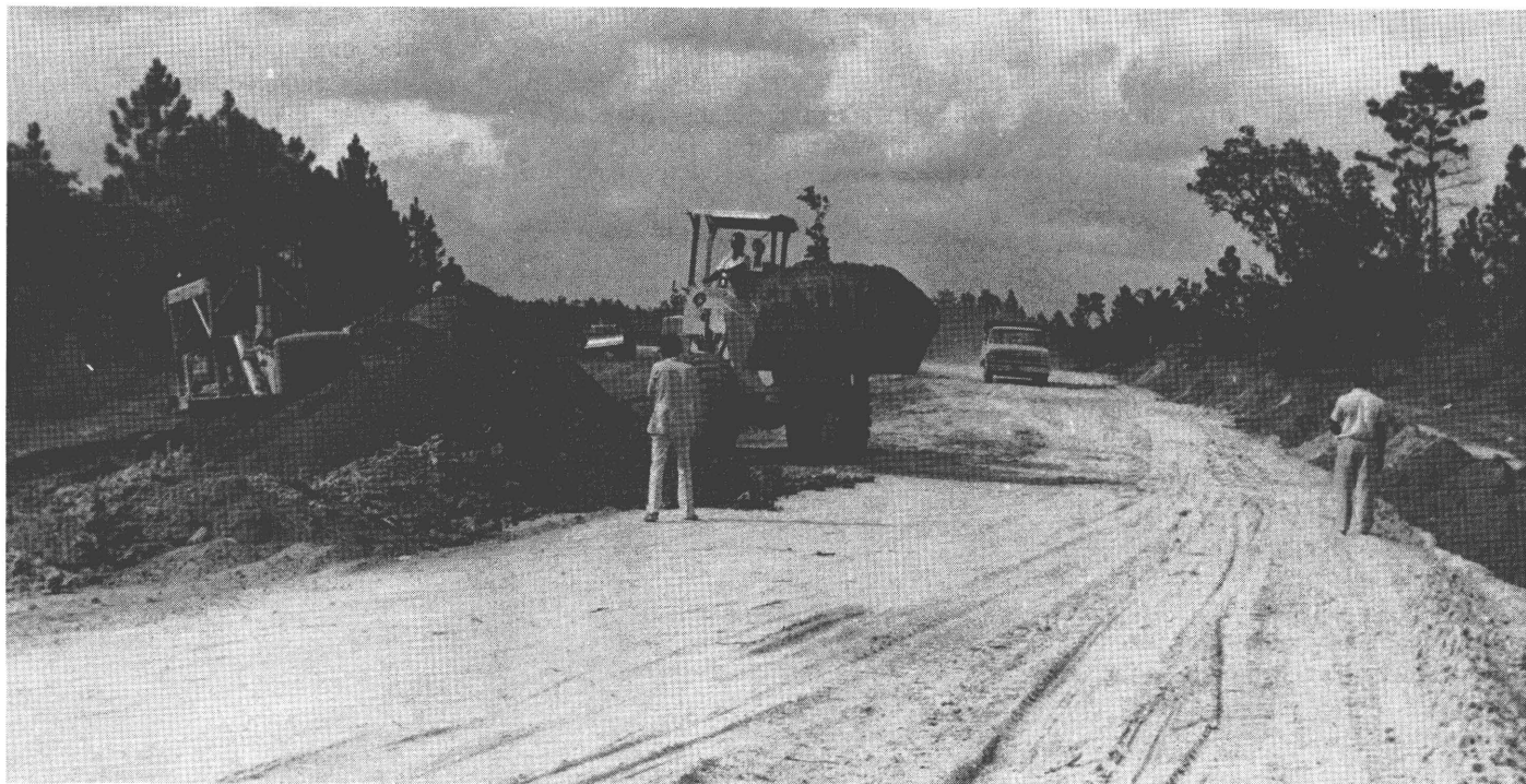
Building work under way on the Western Highway: internal communications are a high Government priority
