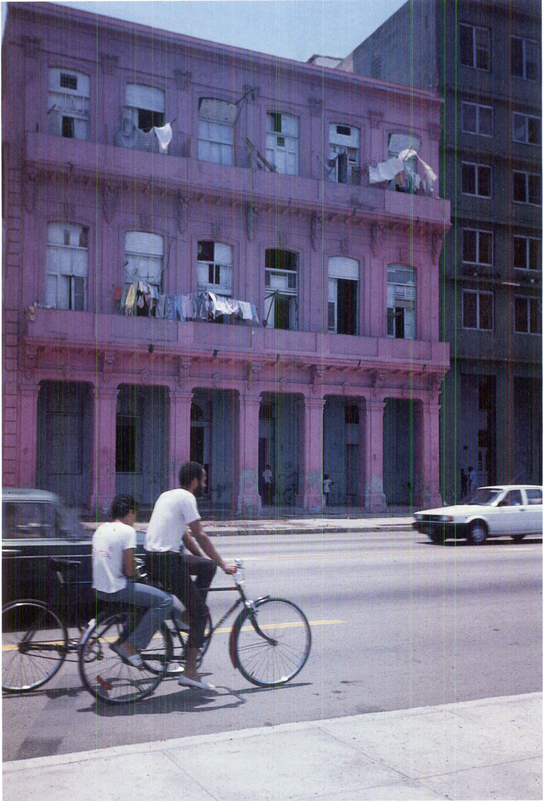
Cuba's economic reconstruction is echoed by the extensive reconstruction of dilapidated buildings
