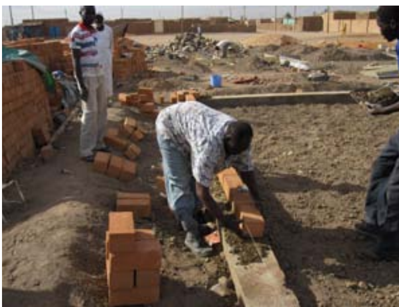
Photo 1 — Building works in the context of the project 'Enhancing the capacity of Khartoum State in the formulation and implementation of urban planning policies' (Sudan)
