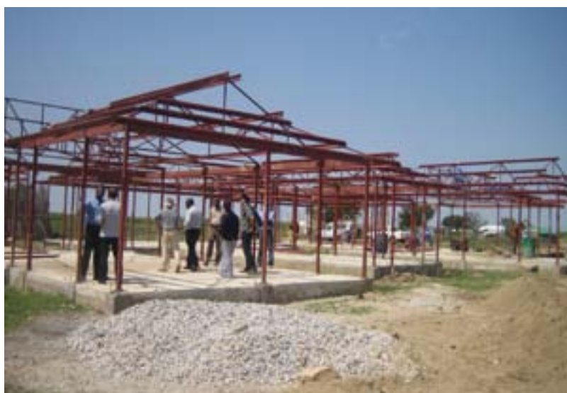
Photo 2 — Construction of offices for the 'Emergency infrastructural support to the Ministry of Legal Affairs and Constitutional Development and the Judiciary of Southern Sudan'
