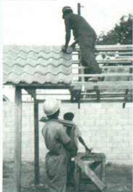
A training exercise in tiling, on a demonstration roof at the Jamaican pilot plant. →
