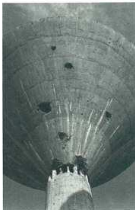
The EDF has financed the rehabilitation of a good deal of the infrastructure, including this water-tower which supplies water to the capital, N'Djamena
