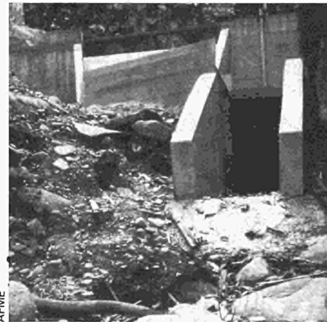
Open channel at the micro-power station of the National Forestry Office in Guadeloupe
