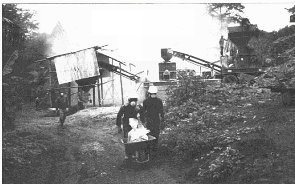
The Lébamba unit. R. to L., the generator, the crusher, with a conveyor belt going straight to the hopper which feeds the grinder, which has its own conveyor belt to the (covered) storage hopper, beneath which is a semi-automatic bagging machine
