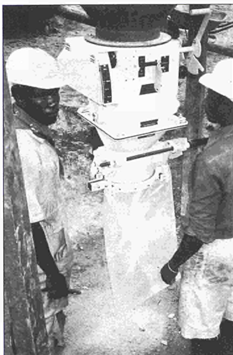
The bagger is regulated to weigh out 50 kg at a time and the flow is stopped automatically as soon as the desired weight is reached
