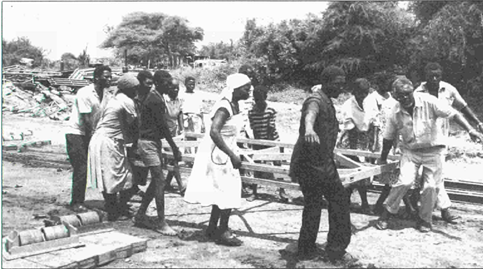
A village community working to install a Bailey bridge — one of the many, highly cost-effective microprojects
