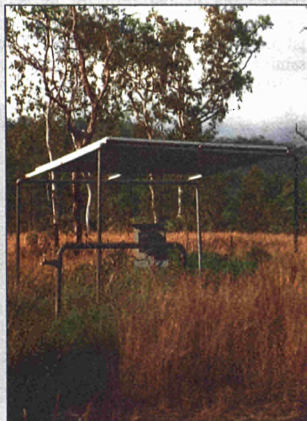
A solar pump supplied by the project
