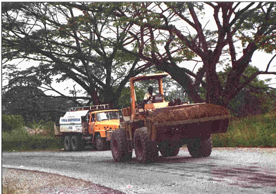
'Roads upgraded to bituminous surface standard' This is on the Brown River — Veimauri road near Port Moresby
