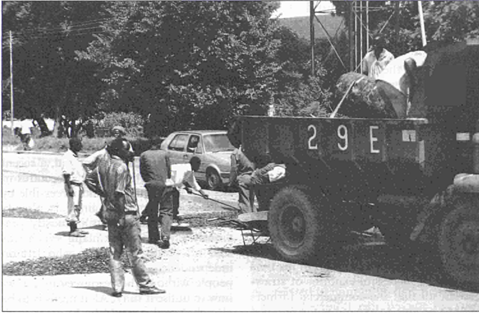
Workers filling potholes in a Lusaka road — a small symbol of the Government's problems. Strapped for cash, it can do little more than patch up the country's infrastructure
