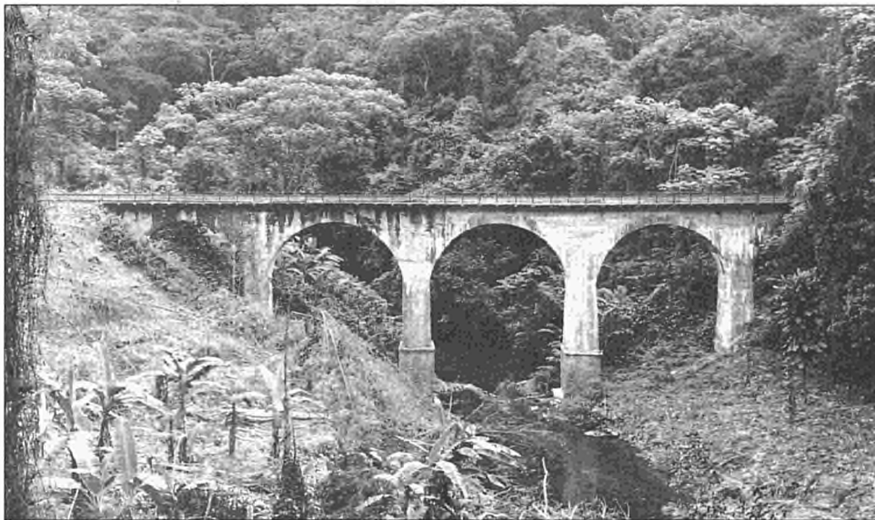
This is a bridge on the vital railway line linking Pointe Noire with Brazzaville in Congo.
