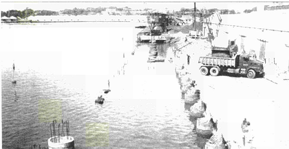
A view of one of the quays at the Port of Takoradi, prior to the completion of rehabilitation works. The Ghana Ports Rehabilitation Project has received substantial support from the European Community
