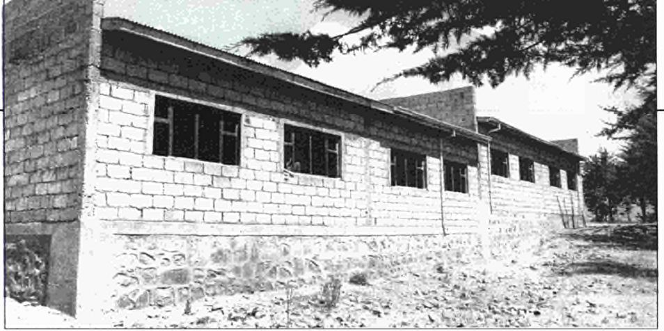
A new rural primary school in Ethiopia nears completion Even capital investments in the education sector usually have a low foreign exchange content
