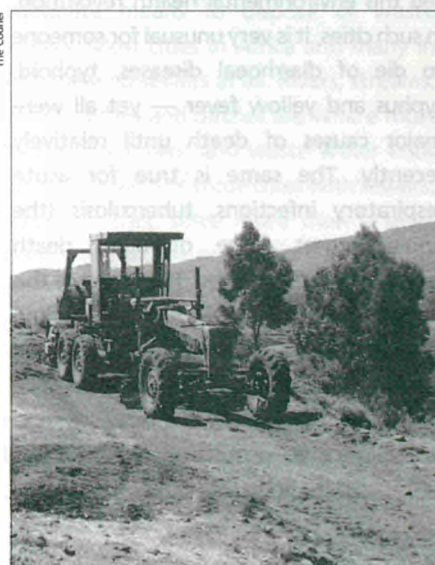
Construction work on a rural road in Ethiopia. 'Improved roads are prerequisites for the healthy functioning of rural-urban links'
