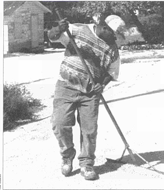
A road in the Family Islands gets a new surface. The government hopes that infrastructure improvements will encourage new tourism investment in less developed islands of the archipelago
