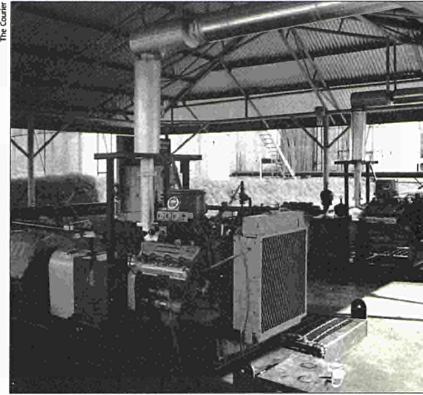
Modern pumping equipment helps to keep the oil flowing
