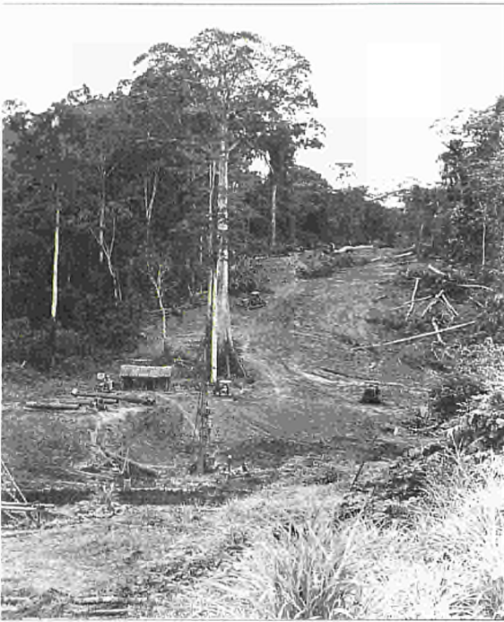
Road-building through the Cameroon tropical forest The government recognised the need for an integrated and long-term approach to environmental management, for the sustainable development of the country's extensive natural resources
