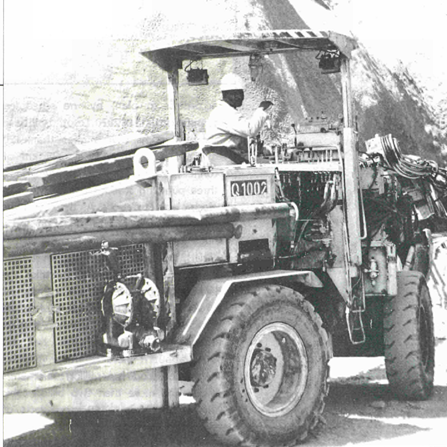
A boring machine about to enter the Muela end of the transfer tunnel
