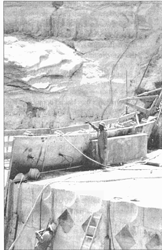
Construction of the Muela tailpond dam, part of the EU supported hydro-electric school
