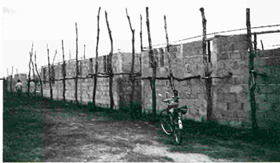
This new EC-funded boarding school, under construction in Guruê, will help make education more accessible to a dispersed rural population.
