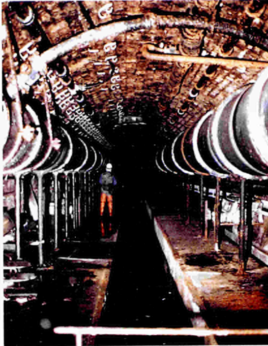
A view of the drainage pipes in the Bordeaux sewage system that will be controlled with the help of the PAYDIRT decision-support system developed in project 5473.
