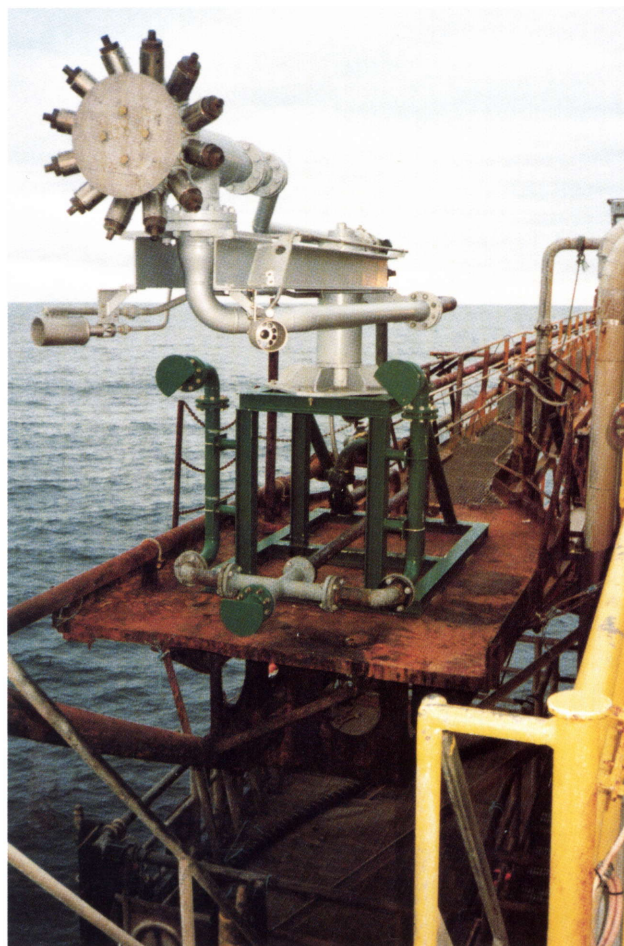
Fig 10 The Evergreen burner installed offshore
