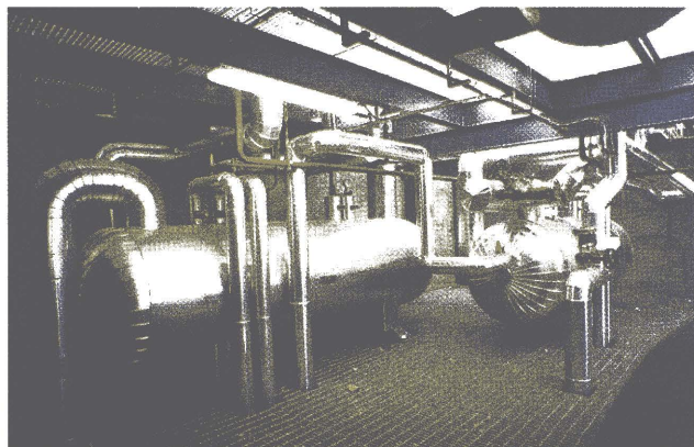
Figure 32. Absorption cooling system
