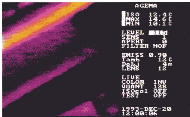
Figure 7. Thermography showing cold losses in a cold storage chamber.
